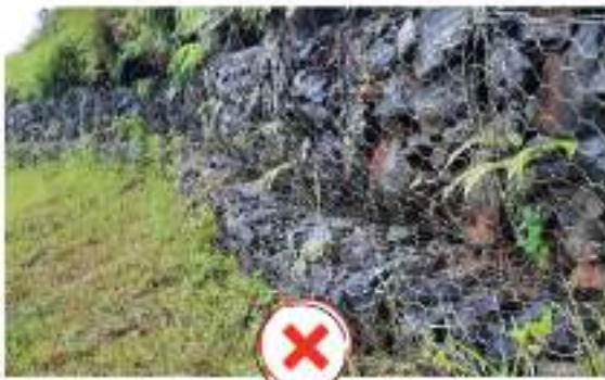
Easy bulging, need more bracing effort
