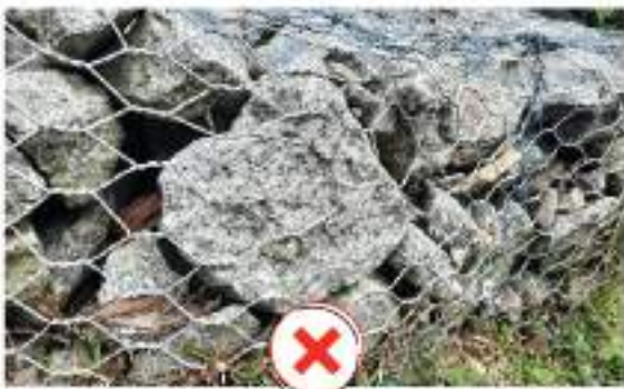
Result to pre-mature failure due to load concentration at single point.
